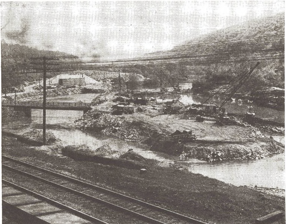
NEW YORK CENTRAL'S ambitious Mohawk River relocation project progresses at a rapid pace. Hazardous curve at Little Falls, N. Y., will soon be a thing of the past
